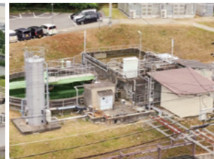
Sakoshi Plant wastewater treatment facility
